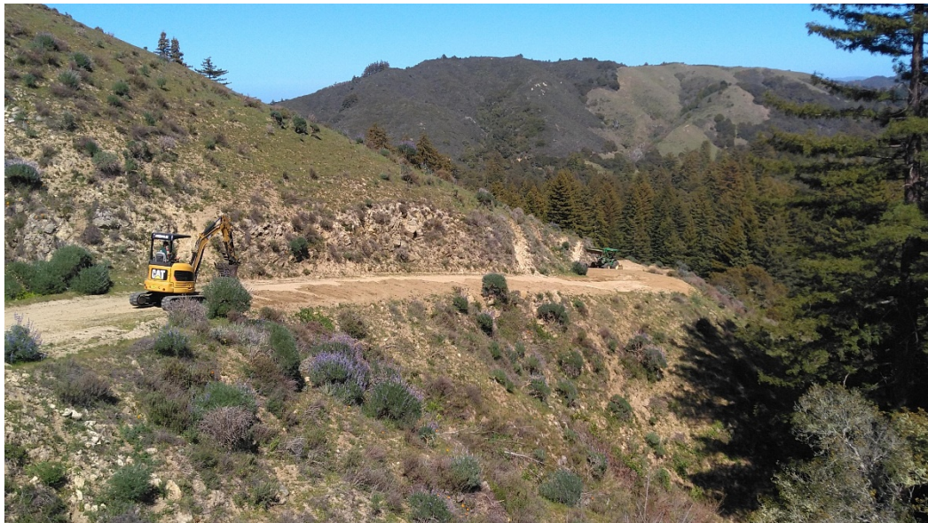
The District's excavator being operated by Ranger Nico In the background, Ranger Jake operates MPRPD's tractor
